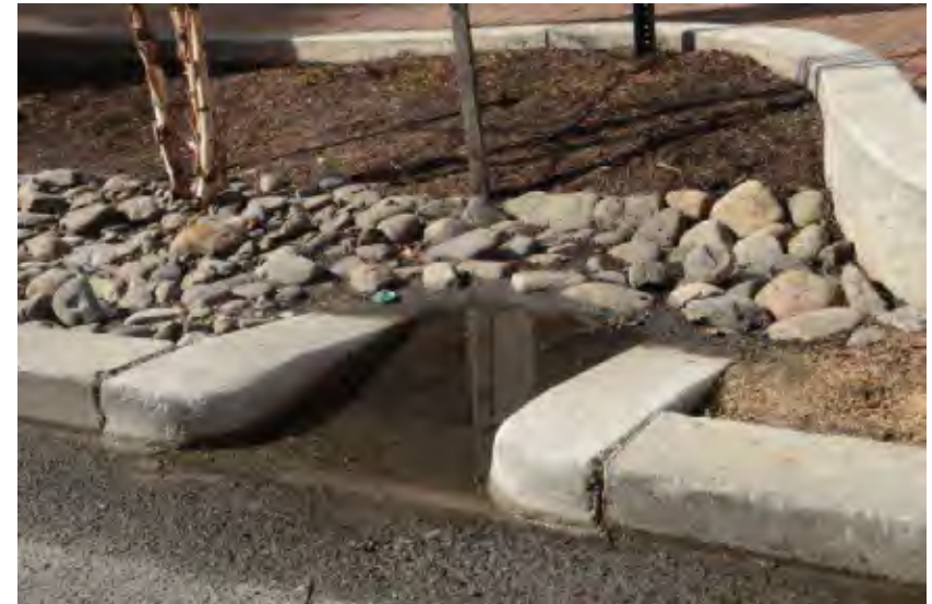
Incorrectly installed inlet.
